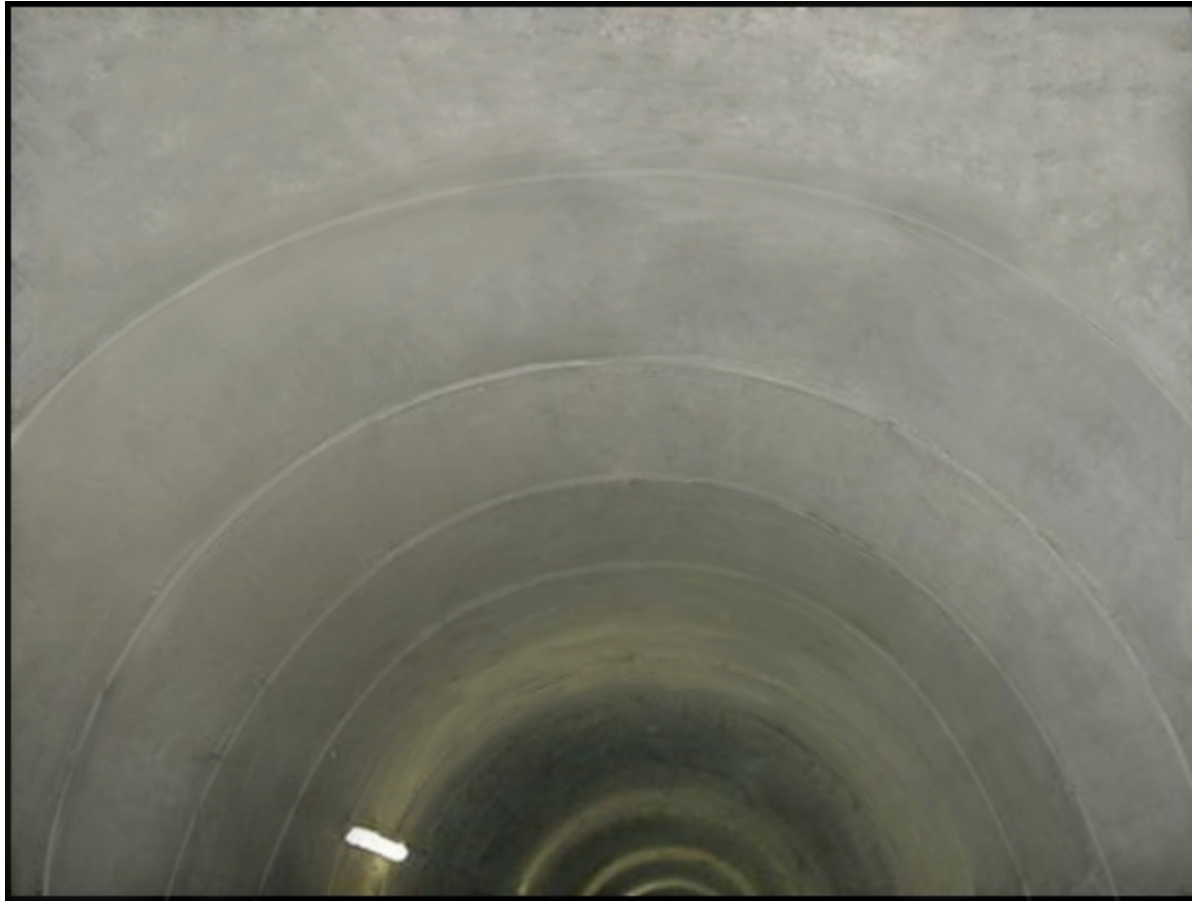
Sanitary Sewer - Tunnel Segments
